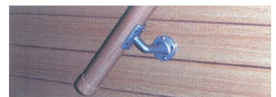
Stairway handrail bracket stop
